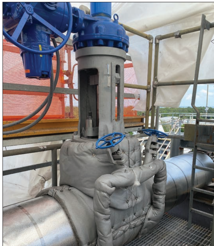
This 14" Class 2500 forged pressure seal valve, installed in a power plant in Florida—part of a large long-term contract with Velan to supply over 100 (12"–24") valves over 5 years.
