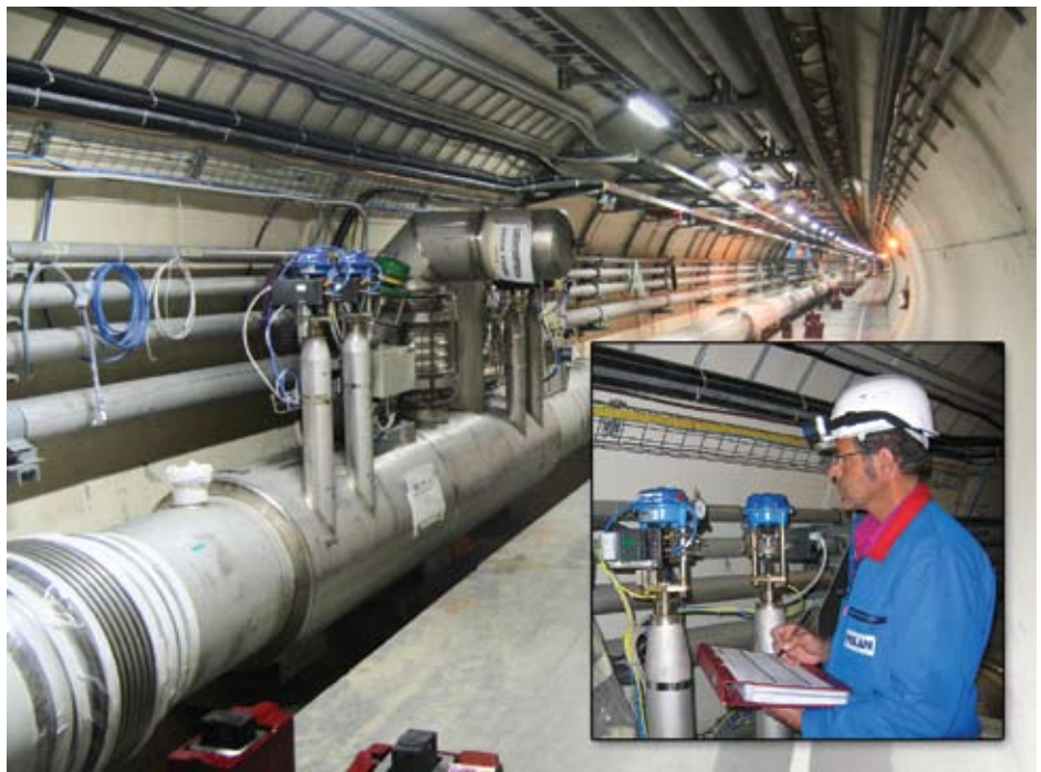
The Large Hadron Collider (LHC) at CERN (European Council for Nuclear Research), Geneva. The LHC is the world's largest, fastest, and coldest accelerator of nuclear particles. Currently, it has over 2,500 Velan bellows seal cryogenic valves installed and controlling the flow of over 700,000 litres of liquid helium.
