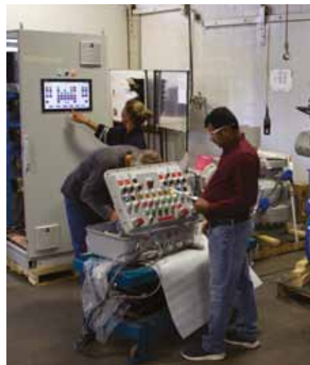
Velan Programmable Logic Controller and control panel
